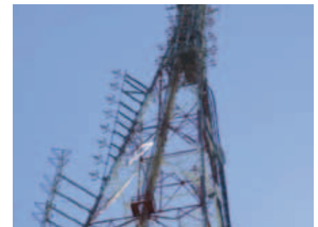
3 FM antennae, one tower. BA Tower Mount Coot-Tha, Brisbane Photo credit: Steve Adler
