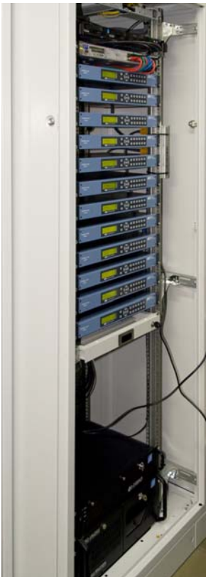
VDL Head-end system at EmiTel in Warsaw
