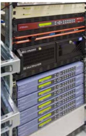
One of the two VDL head-end systems at Bayerischer Rundfunk in Munich
