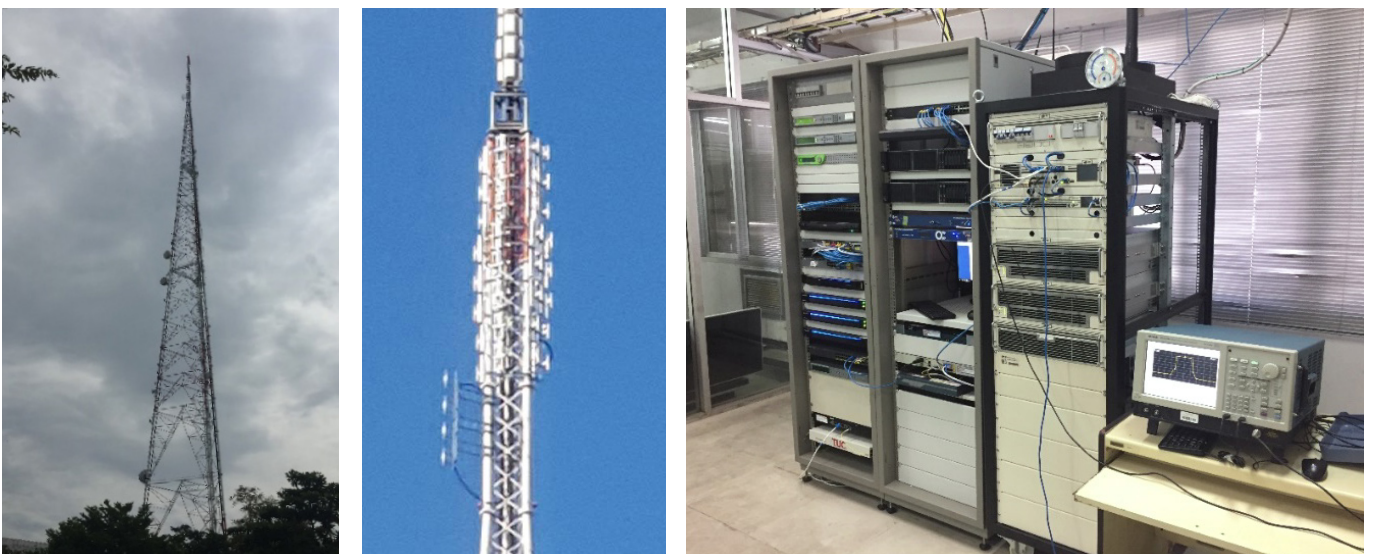
Figure 5-2: Example high-power DAB+ demonstration system
