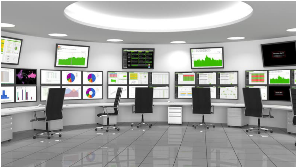
Figure 10-1: A modern Network Operations Centre 84
