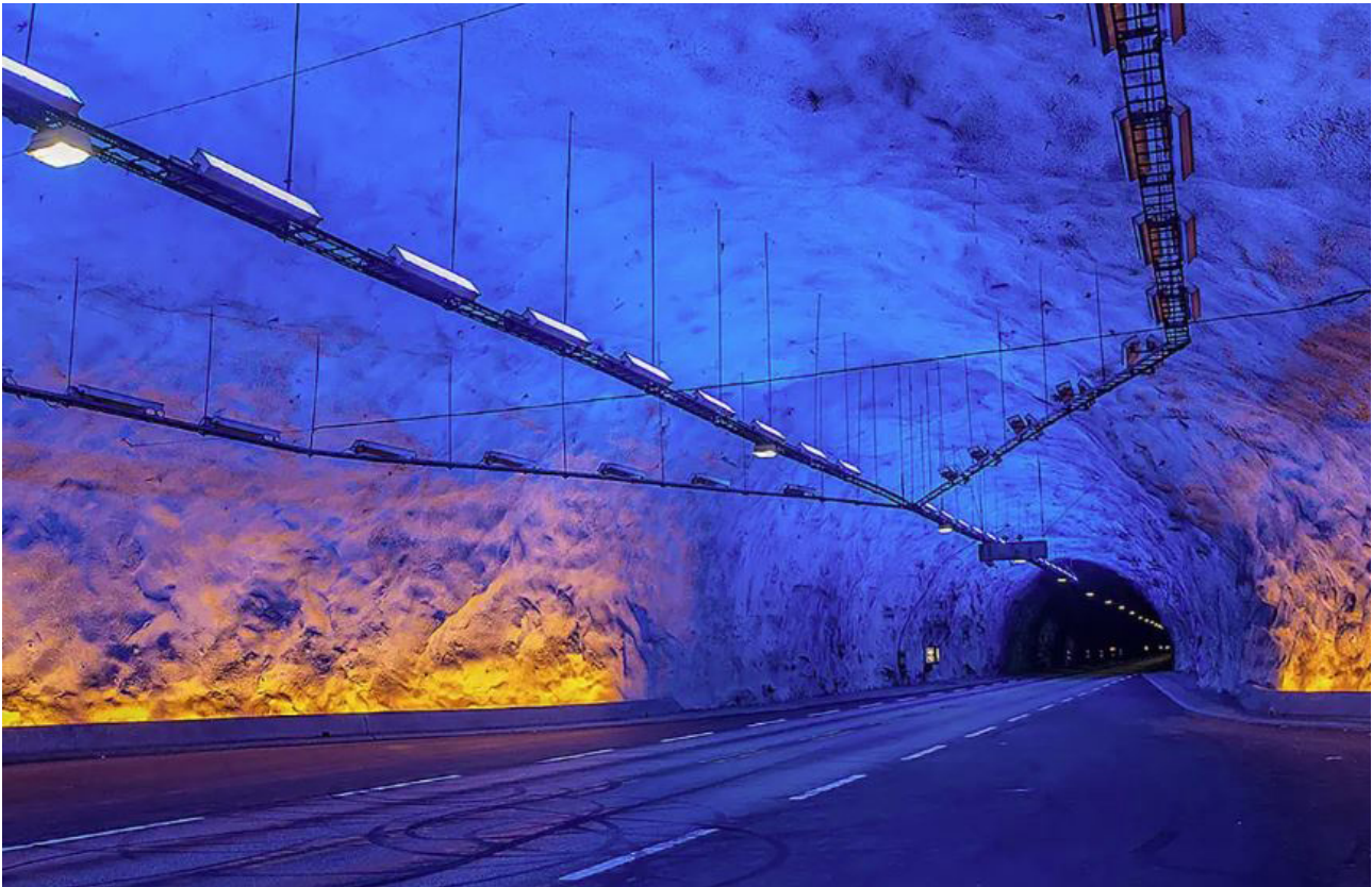
Figure 8-30: Example infrastructure in a road tunnel which includes power distribution, lighting and communications via leaky feeder coax systems 60
