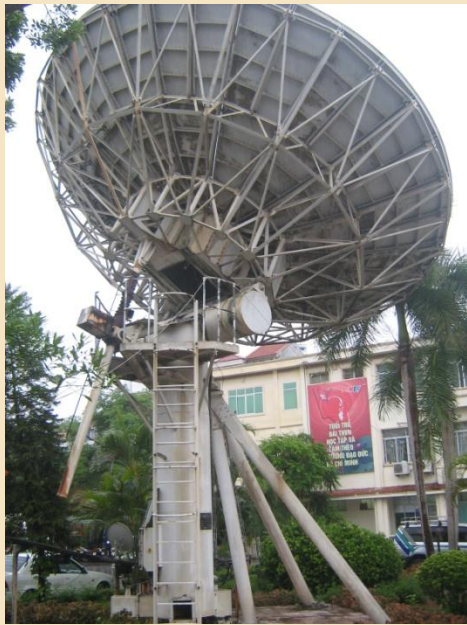
Uplink antenna for DTH
